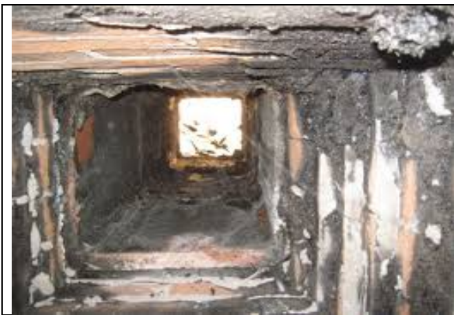
Chimney Refurbishment - Before Old chimney is coated with soot and structural strength is significantly reduced due to heat or damp damaged, weak mortar.
