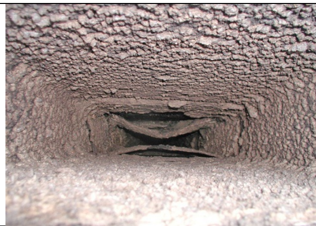
Chimney Refurbishment - After Old chimney is sprayed with LightCem SPRAYFAST which penetrates mortar joints and thereby significantly strengthens structure. Sleeve can then be fitted and additional SPRAYFAST can be poured in to solidify whole structure.
