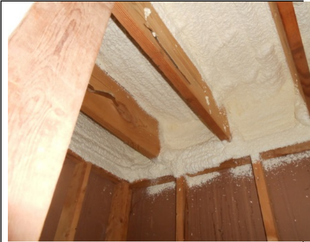
Fire Protection Coatings LightCem FIRESHIELD was applied to vulnerable areas to enhance fire-protection.
