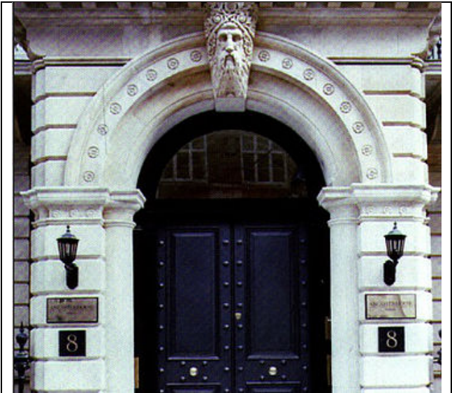
Queen’s House – Leicester Square Repairs to main Façade using LightCem LITECRETE - still in perfect operational condition after 20 years.
